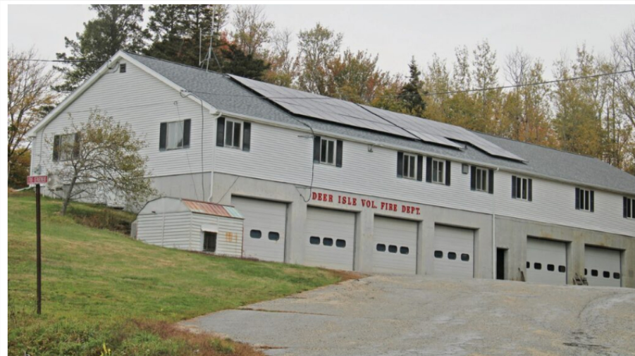
Solar panels have been installed at the Deer Isle town hall. Switching the building to solar power is part of a months-long effort by Deer Isle and Stonington, who both received a grant to outfit solar panels on town buildings. Deer Isle Town Manager Jim Fisher said the panels are in place and the accompanying battery storage systems are set to be installed in the coming weeks. BY WILL ROBINSON
